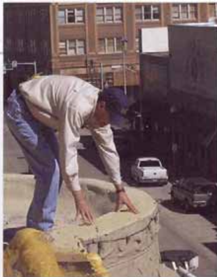
Part of an inspection team, engineer Steve Lucy checks the roof of a commercial building in downtown Lake Charles, La.
